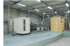
▲補機類 Auxiliary machines
