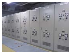
▲高圧発生盤 High-voltage generator
