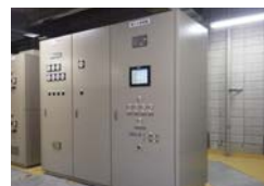
▲集じん制御盤・補機盤 ESP control panel and distribution panel
