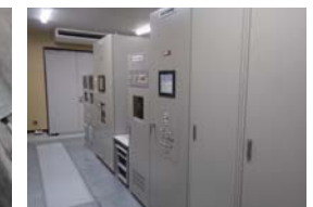
▲計測制御盤 Measurement control panel
