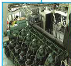
Control panel and TRO meter
